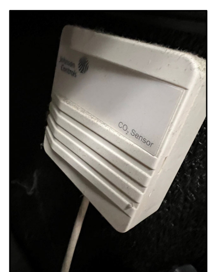
3 TYPICAL UNIT MOUNTED CO2 SENSOR M-701 NTS
